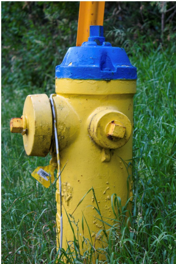
Figure 11. Fire hydrant painted according to the NFPA 291 colour code.
