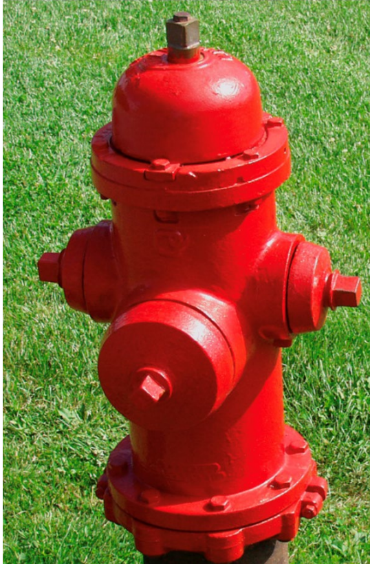
Figure 12. Example of a private fire hydrant.
